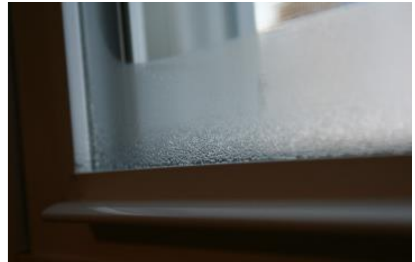
Condensation on windows
