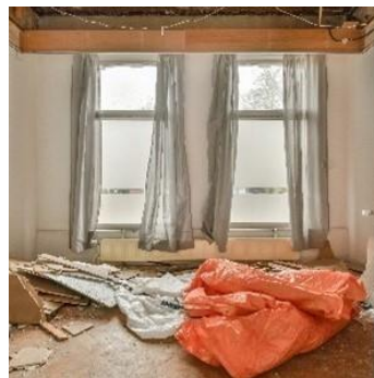
Rooms being in disrepair
