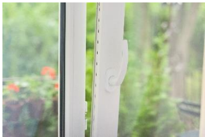
Difficult to open or close
