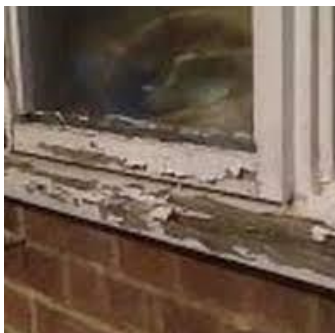
Flaking paint or signs of rotted wood
