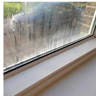
Condensation trapped between the windowpanes
