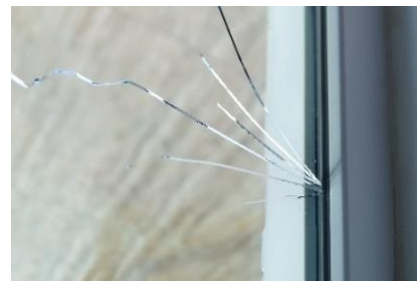
Broken or cracked glass
